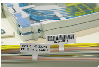
Fibre optic cable markers
