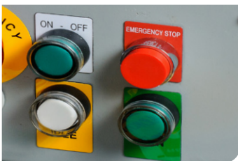
Control panel labels
